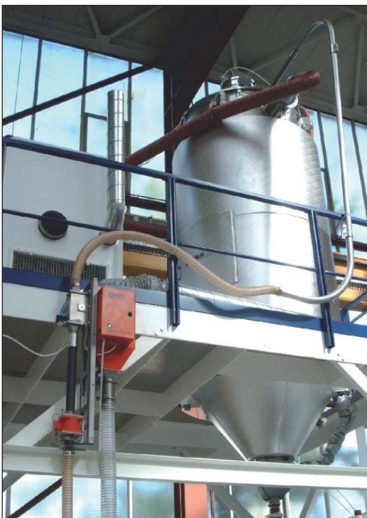
GF metal separator installed in vertical pipes
